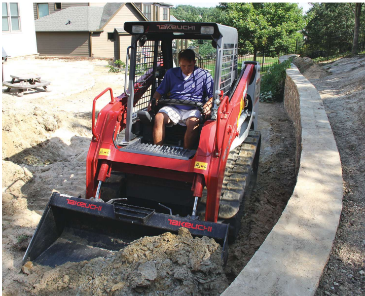
With flat building spaces quickly becoming extinct, retaining walls have become a popular request from customers.
